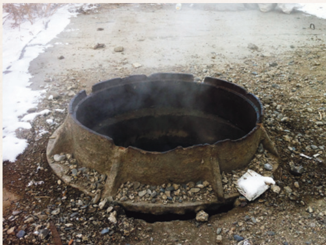
An open manhole in UB, Mongolia which shows someone has often passed through it
